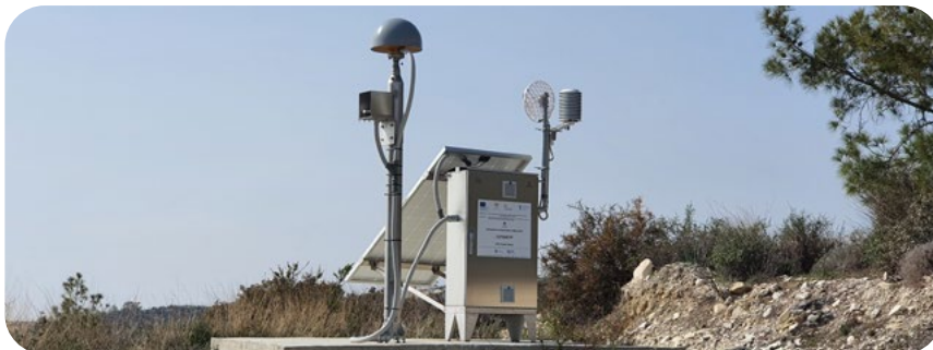
Natural Hazards Monitoring & Prevention System - CyCLOPS
