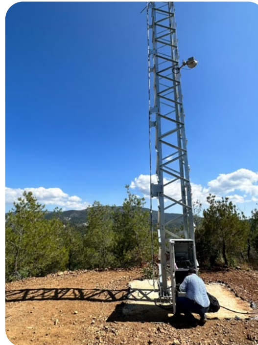
Fire early warning system in Cyprus
